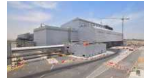
Dubai Waste Management Centre
