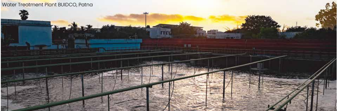
Water Treatment Plant BUIDCO, Patna
