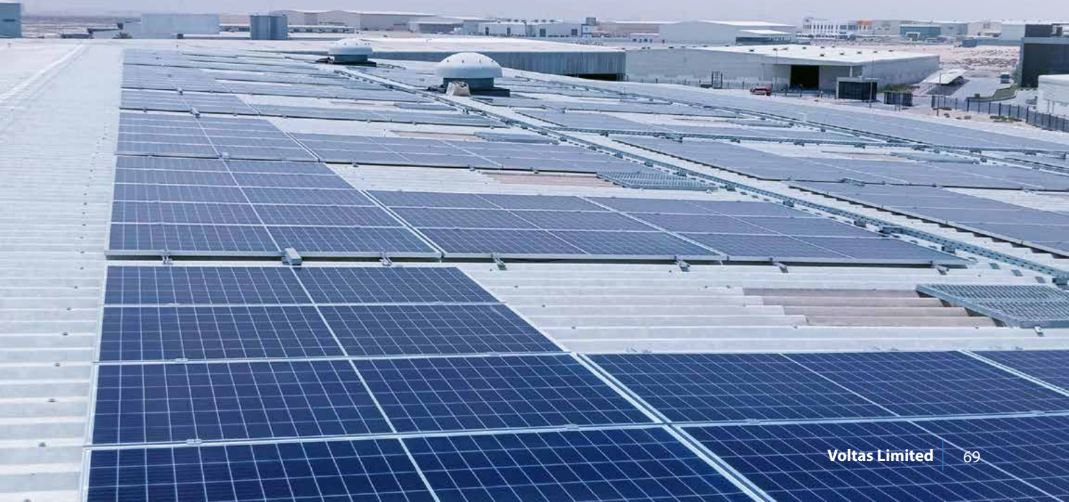
Solar Panels at our Factory
